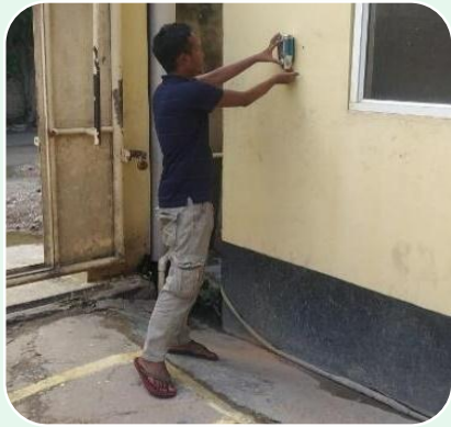
Hand sanitizer installed at entrance
